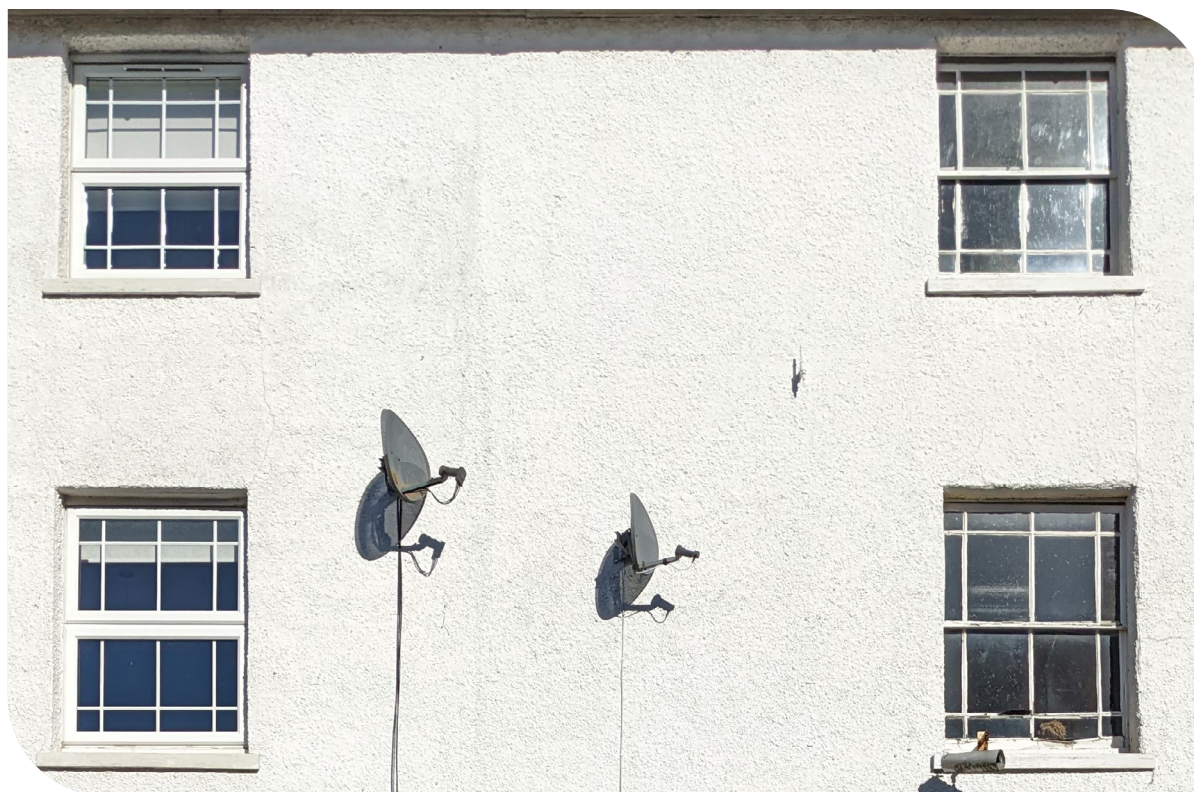
Historic timber sash window, right, and replacement uPVC windows, left. The pebble-dashing and satellite aerials are also non-traditional elements that harm character and appearance
