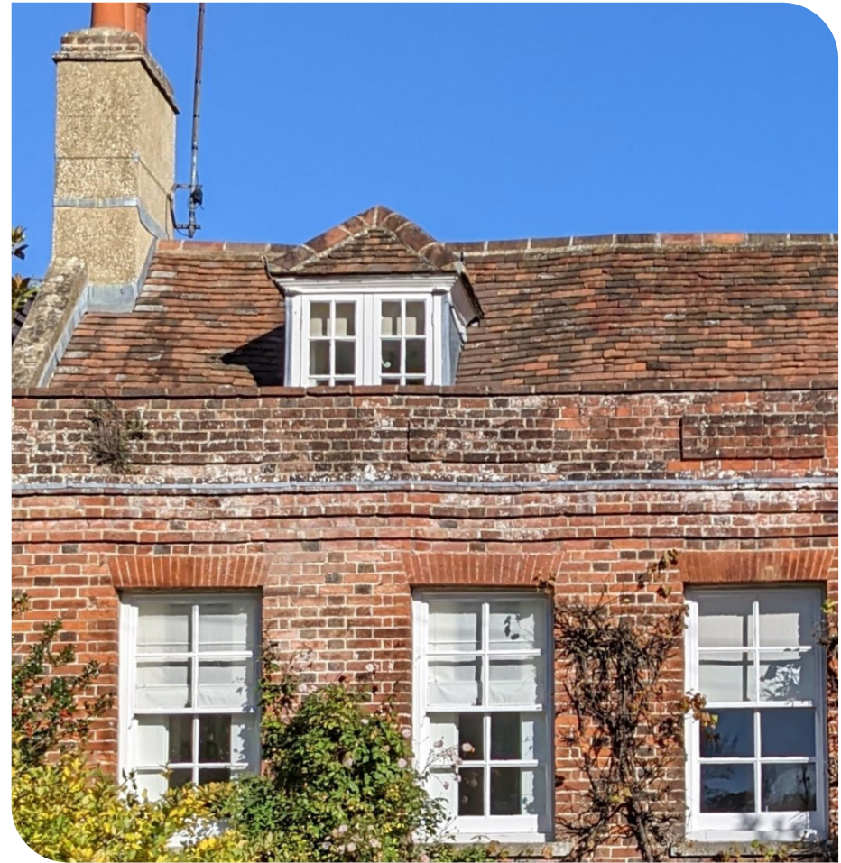
Kentish 'peg tiles', irregular roof line and dormer window. Traditionally, where they are used, dormer windows are small and visually subservient
